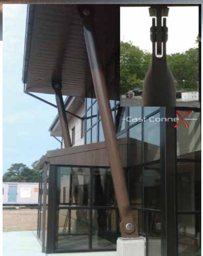
Cast ConneX® Universal Pin Connectors™ employed at both ends of the architecturally exposed, inclined steel columns supporting a roof overhang at the New Jersey Air National Guard Operations and Training Facility, Egg Harbor, NJ. Courtesy of Carlos de Oliveira, Cast Connex Corporation.
