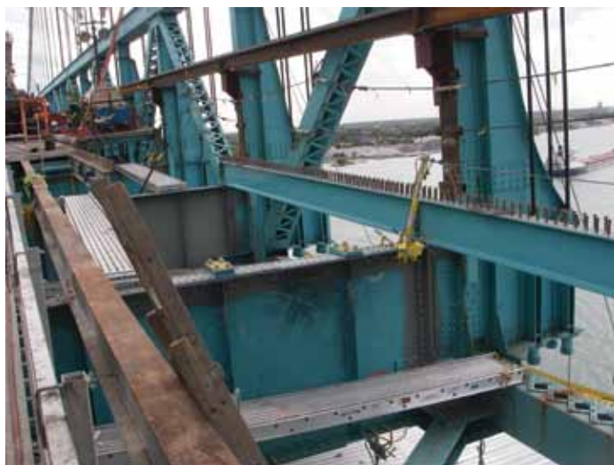
Deck replacement of the suspended spans included installation of new steel stringers.
