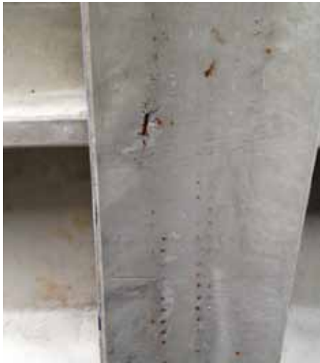
Figure 4 (from Part 1, Sept. 2013): Rust staining due to internal corrosion of post-tensioned girder reinforcing.
