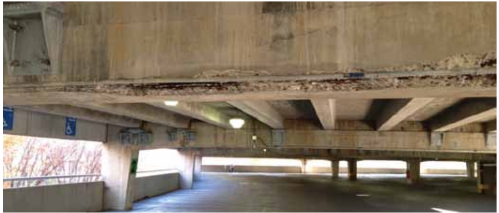
Figure 2 (from Part 1, Sept. 2013): Spalling due to deteriorated strands at precast girder.
