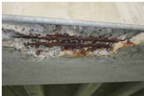
Figure 3 (from Part 1, Sept. 2013): Corroded and failed prestressing strands at precast girder.
