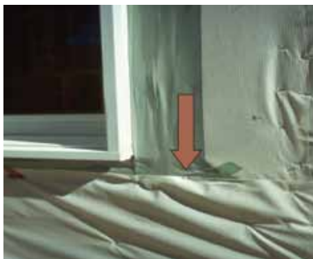
Figure 6: Reverse flashing at window.
