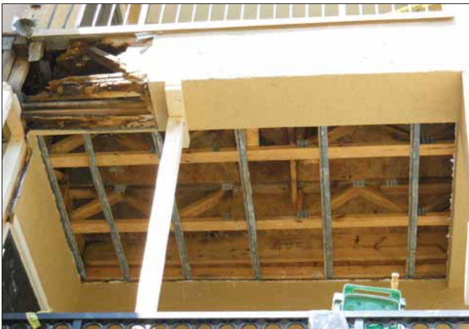
Figure 4: Decay at balcony edge where inadequate drainage provided led to decay.
