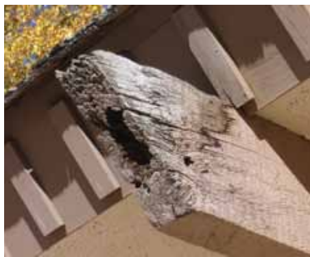
Figure 7: Untreated wood beam with exposed end grain.
