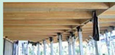
The Promega biotechnology production facility features an innovative mix of glued laminated timber and cross laminated timber.
