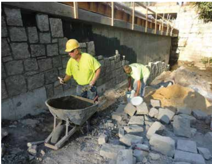
The refurbished bridge used stone facing over the wingwalls and black metal fencing to create a similar aesthetic
