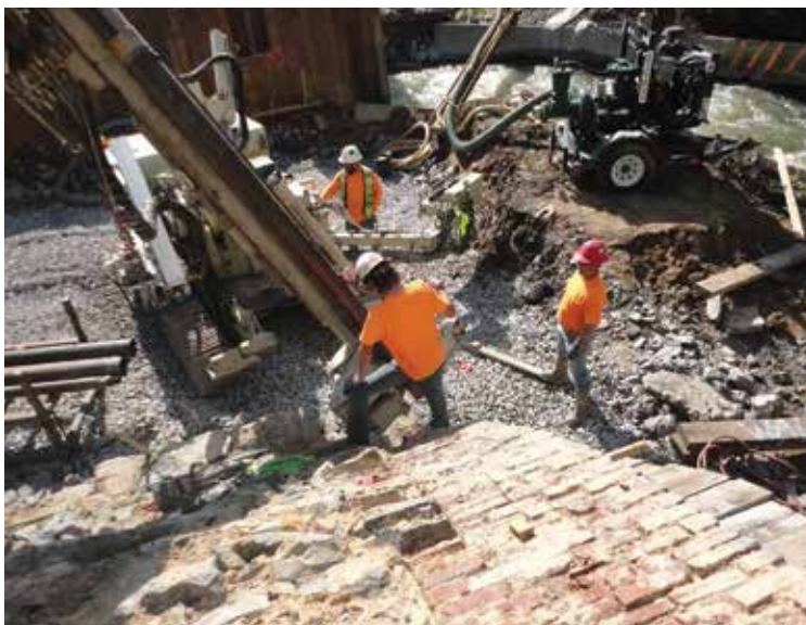
Burgess & Niple designed the bridge with micropiles instead of hammer-driven piles to reduce vibrations adjacent to the existing stone masonry.
