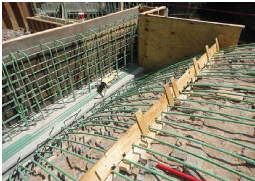
A new reinforced concrete arch was designed and placed over the top of the existing arch to provide full live load capacity.
