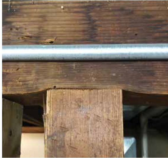
Figure 3. Deformation at beam bearing.
