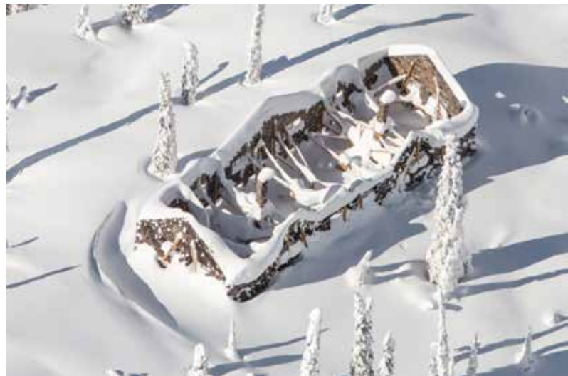
Figure 1. The chalet survives the first winter after the fire, thanks to emergency bracing. Courtesy of GravityShots.com.
