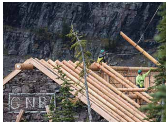
Figure 5. Timber framers set the log rafters via helicopter assist. Courtesy of A Boring Photo.
