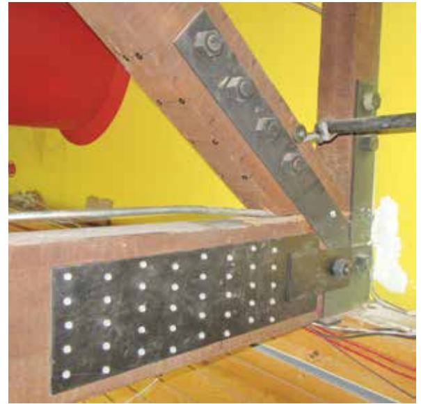
New heel plate connection at the bottom chord and supplemental HeadLOKs installed on the diagonal bottom surface.
