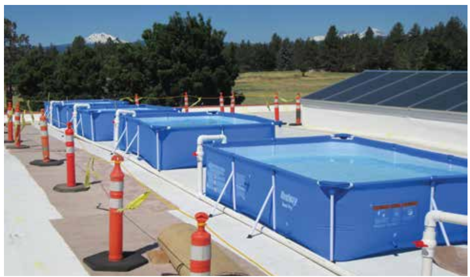
Pools filled with water on the roof during load test of the repaired truss.
