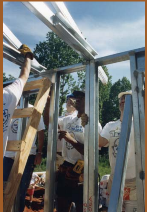
Proper attachment of the truss system to the structure is essential, especially in areas of high uplift loading.
