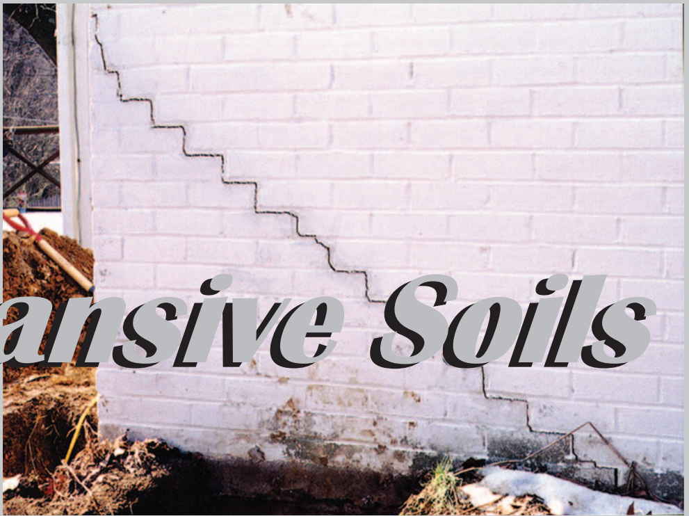
Stair step cracking in brick veneer
