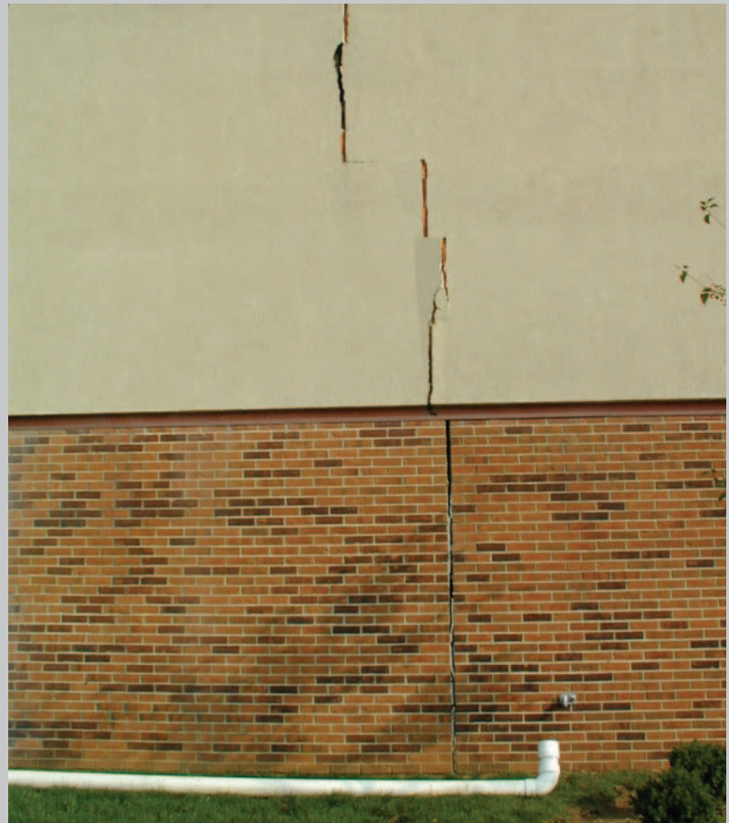
Stair step cracking in brick veneer
