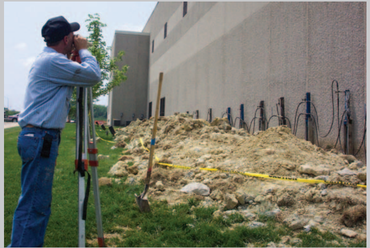
Commercial office building foundation failure
