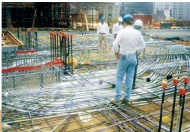
Not coordinating the conduit placement with the Electrical Engineer can cause a problem!
