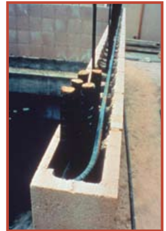
Severe congestion of reinforcement required the facespalls of this concrete masonry wall to be cut to accommodate the steel. Such congestion should be avoided for economy, and to ensure proper placement of grout around the reinforcement. Photo courtesy of Phillip Samblanet.
