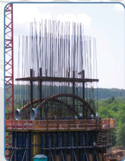
The first two cradles were positioned in the seventh lift on each of the pylons on July 18 th , 2005.
