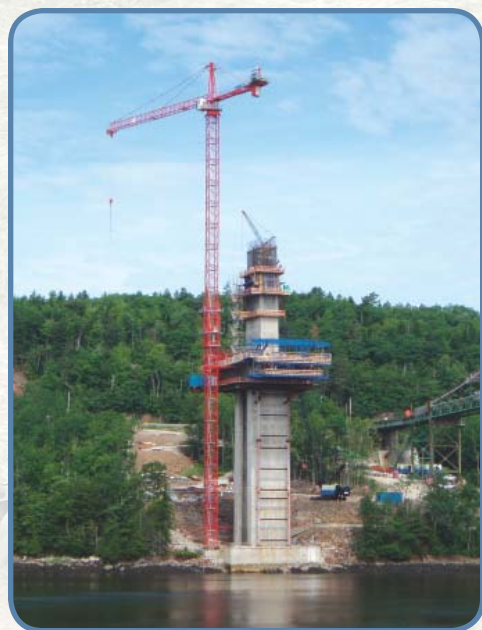
The western pylon, adjacent to the Fort, is being cast in 16 lifts from deck level to the base of the public observatory, located at elevation 389 feet.
