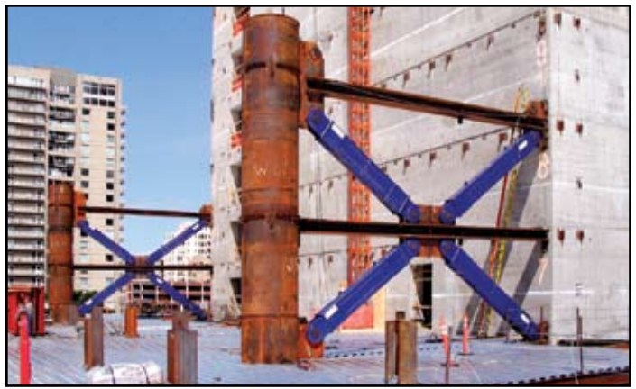
Figure 5: Buckling-restrained braces connect the core to concrete-filled pipe columns and, through the action of steel yielding within concrete confinement, act as a "seismic fuse" during an earthquake, absorbing energy and preventing damaging to the rest of the structure.
