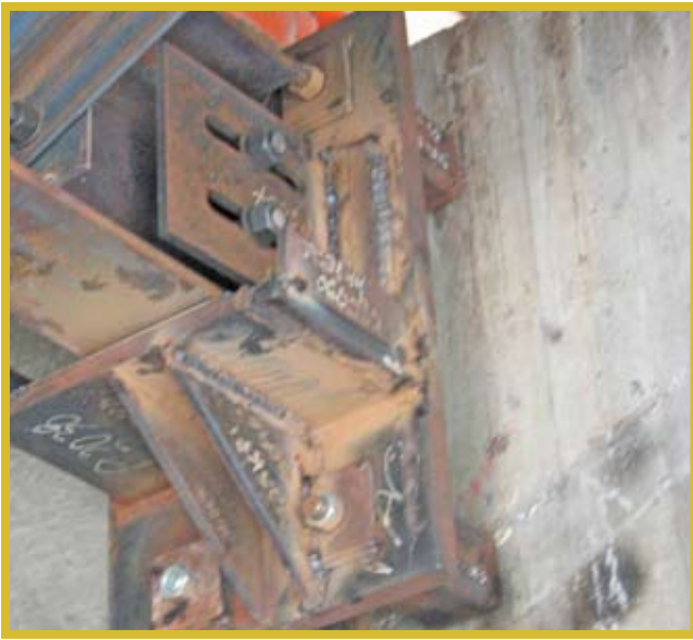
Figure 4: Multi-Directional Slide Bearing of new suite tower beam to existing concrete column to transfer gravity loads only.
