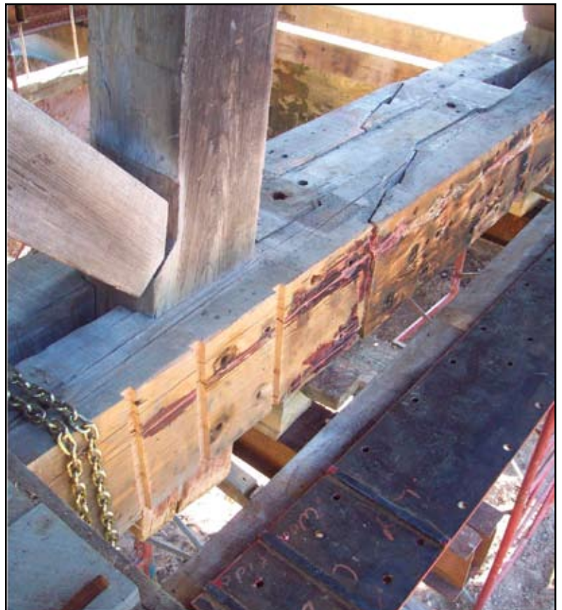
Figure 7: Scarf splice in lower chord. Keyways have just been cut in wood to match those on new side plate. Timbers that loosened when sag was jacked out were resealed and shimmed.
