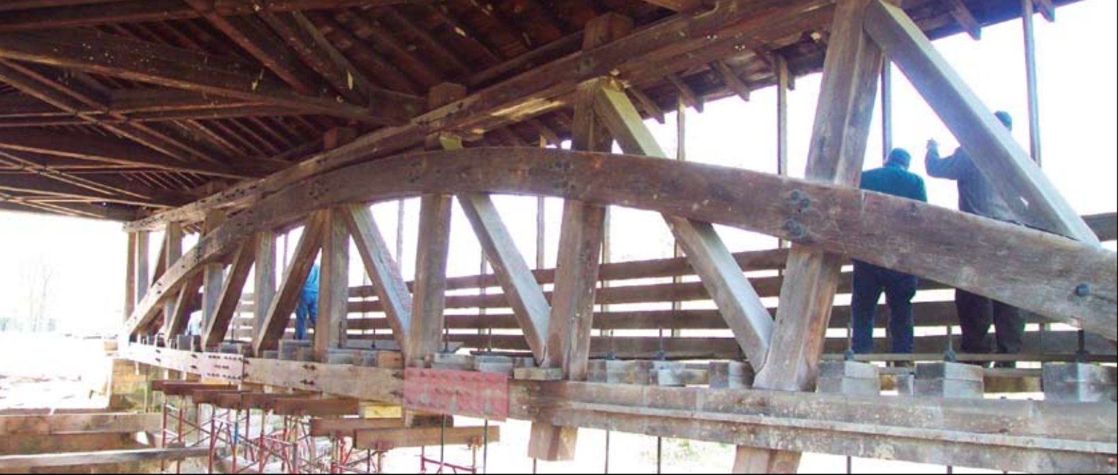
Figure 6: IDNR engineers inspect the shored, but not yet jacked, trusses. They are standing on the walkway for the tow horses.
