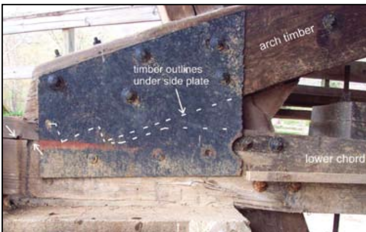
Figure 4: Typical bearing seat. Thrust from arch sheared top of lower chord, splitting a bolt hole (arrows). Lower chord crushed and curved as it passed the face of abutment.
