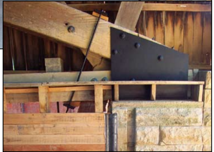
Figure 8: Bearing seat area, new flume, and expansion joint seal after repairs were completed.
