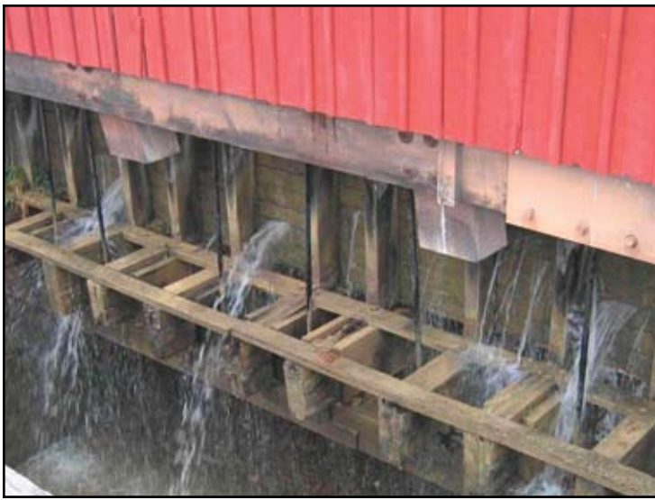
Figure 3: Leaks in the flume caused decay in its supporting structure.
