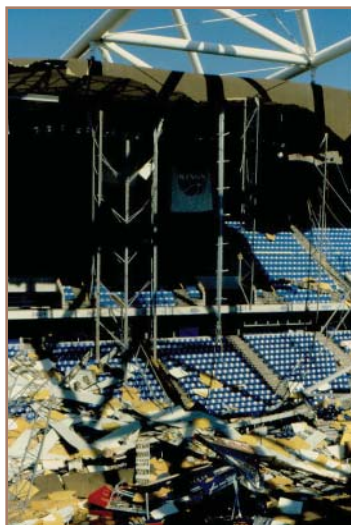
Kemper Arena Roof Failure, Kansas City, MO (1979).
