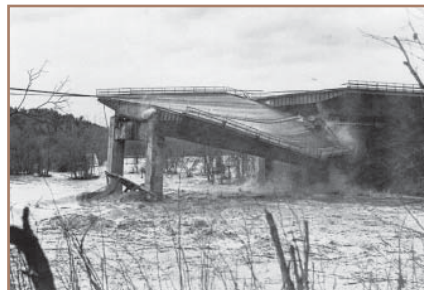
Schoharie Creek Bridge failure (1987).
