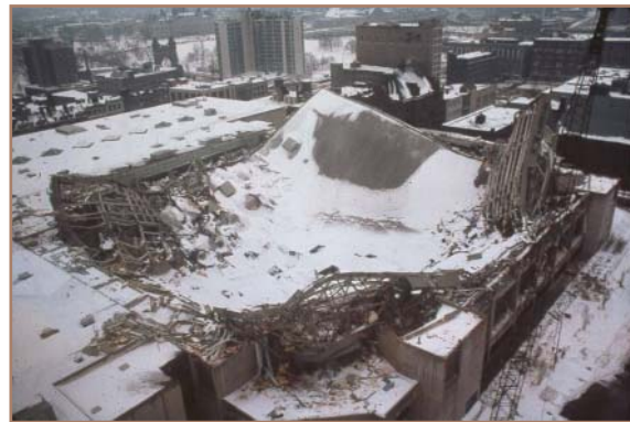
Hartford, Connecticut Civic Center Collapse (1978).
