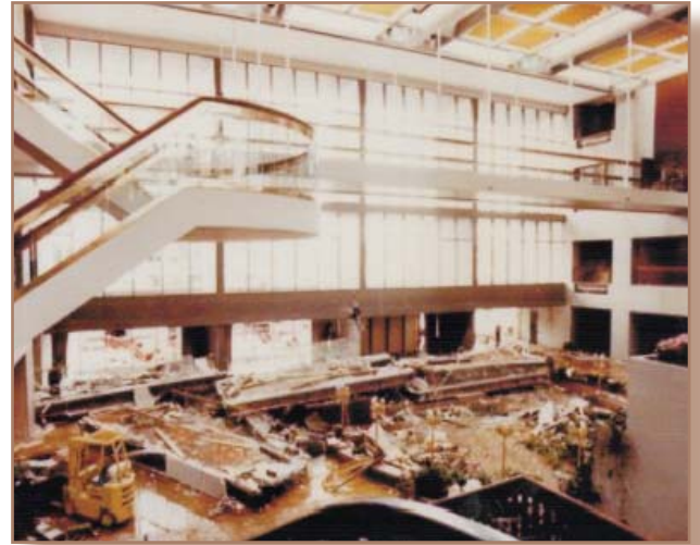
Kansas City Hyatt Regency Hotel walkway failure (1981).
