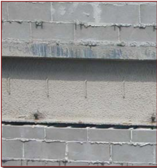
Figure 15: Locate bond beam directly under steel beam only if there is room to grout from the exterior side
