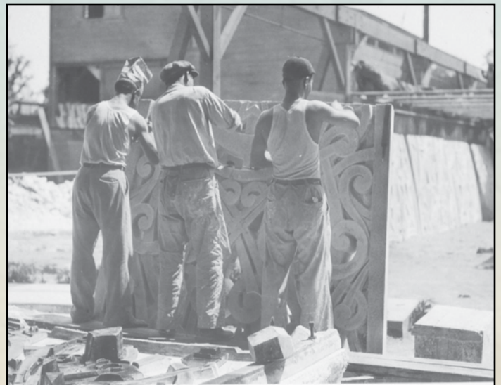
Due to the requirements of the finish, several workers at one time were required to wire brush the panels to expose the quartz aggregate prior to the green concrete setting
