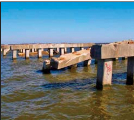
Figure 4: Destroyed US 90 Bridge over St. Louis Bay
