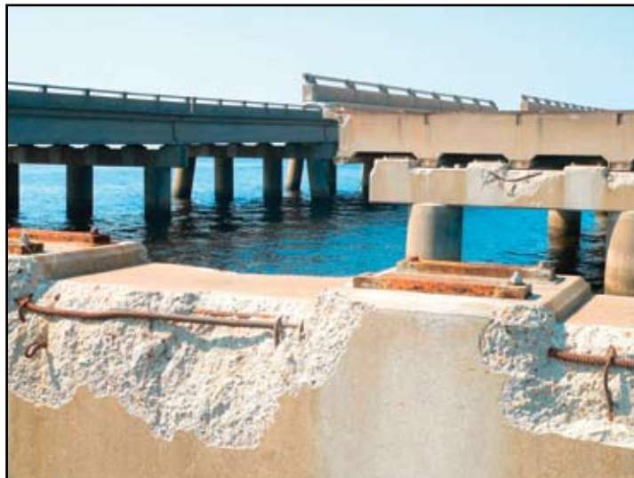
Figure 2: Failed Anchor Bolts and Shifted Spans
