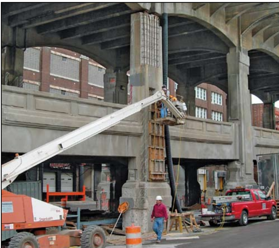
Concrete repairs completed prior to installation of ECE treatment. Courtesy of Vector Corrosion Technologies.
