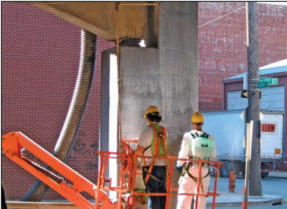
Application of concrete sealer to prevent future chloride contamination after ECE treatment is completed. Courtesy of TranSystems.
