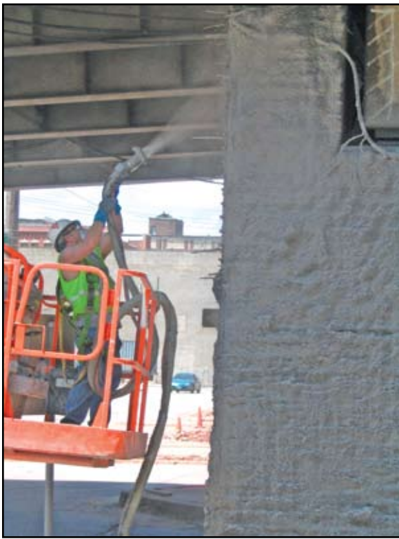
Application of cellulose fiber for conductive media around temporary anode. Courtesy of TransSystems.
