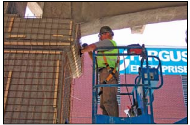
Installation of temporary anode mesh onto concrete surface. Courtesy of Vector Corrosion Technologies.
