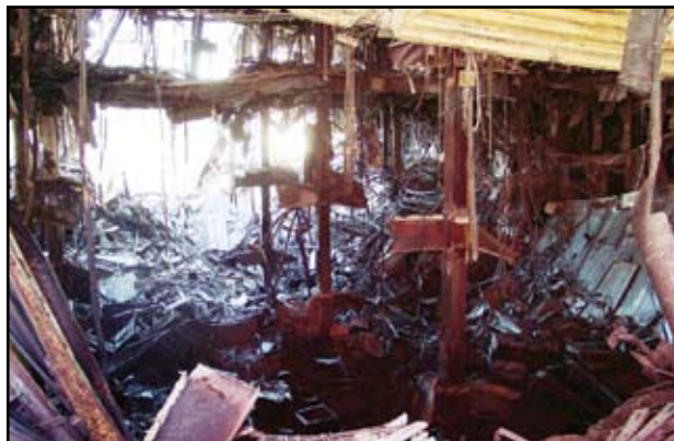
Figure 1: Partial Collapse of WTC 5 [FEMA, 2002]
