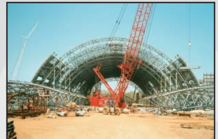
The site assembled center portions are craned into position completing the arch. Additional assembled lower, side portions which have not yet been raised are visible in the foreground on either side of the crane.
