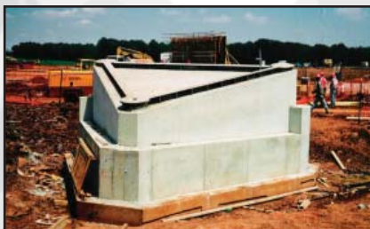
The completed foundation block stands ready for erection of the arch truss. The architecturally exposed upper portions of these concrete bases are a visual feature in the main hangar.
