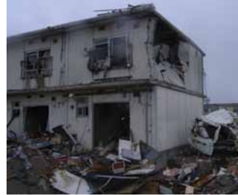
Figure 6: Ian Robertson of the ASCE Tsunami Reconnaissance Team Examines the Results of a Tsunami Bore-Projectile Car Impact on a Structural Precast Bearing Wall Apartment Building in Yuriage, Natori.
