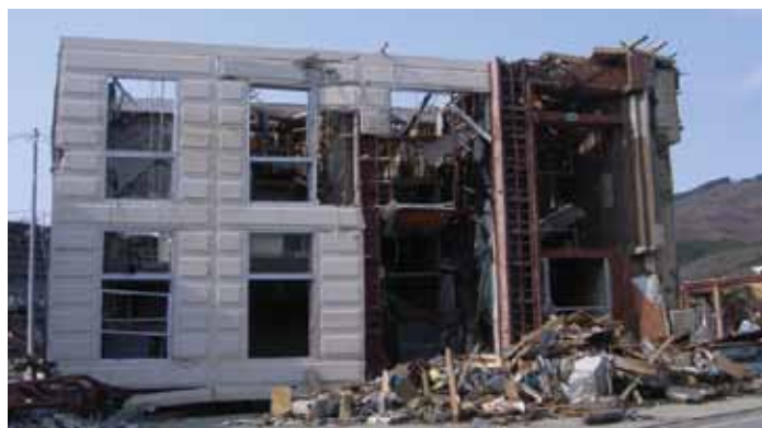
Figure 2: Overturned Steel-Framed Office Building in Onagawa.
