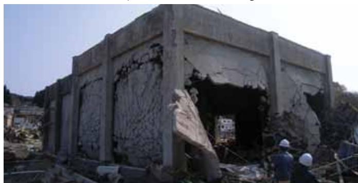
Figure 3: Onogawa Reinforced Concrete Building Frame Structure with Shear Wall Blow-outs.
