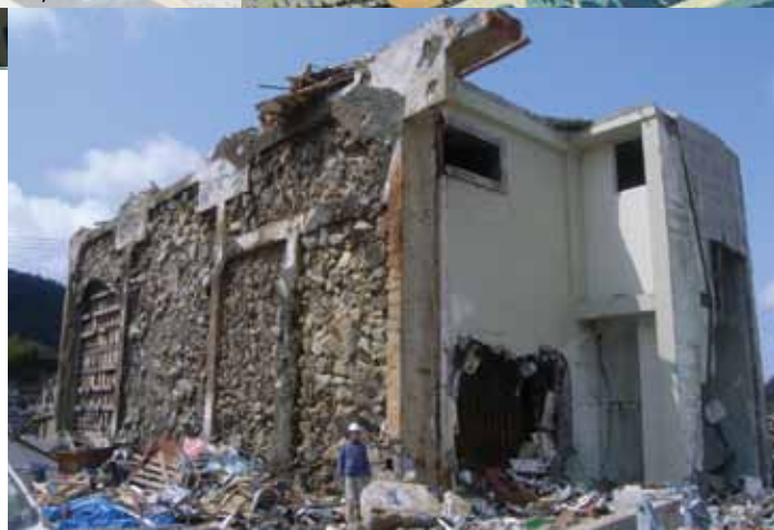
Figure 1: Overturned Cold Storage Building in Onagawa.
