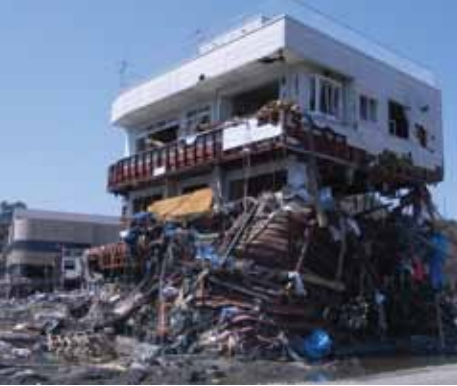
Figure 4: Otsuchi Town Three-Story Steel Moment-Resisting Frame with 15-foot tall Enwrapping Debris Load.
