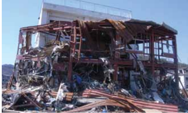
Figure 5: Otsuchi Town Collapsed Three-Story Steel Moment Resisting Frame with Debris Load.
