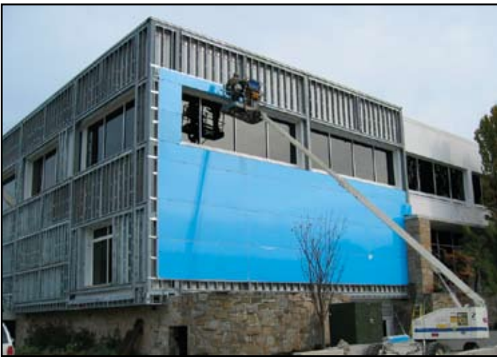
Welded Steel tube system has been installed and supported at the base. Cold formed metal stud framing and new facade installation is in progress.
