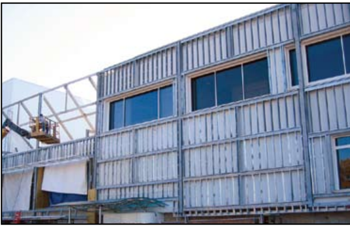
In order to resist the wind loads the front entrance welded steel tube framing had to be braced back diagonally to the existing roof framing.
