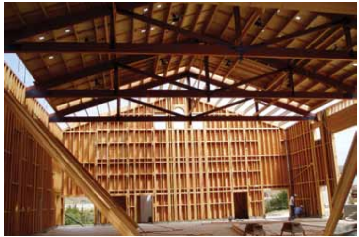
At Cayucos Elementary School, the roof is made from custom glulam trusses. Courtesy of RRM Design Group, Taylor & Syfan Consulting Engineers.
