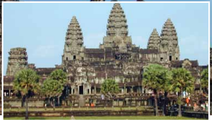
Figure 1: Conservation of the stone roof structure being conducted by the World Monuments Fund at the "Churning of the Sea of Milk" gallery, Angkor Wat, Cambodia. Courtesy of the World Monuments Fund.
