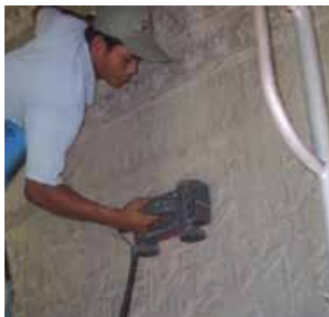
Figure 2: Khmer technician using microwave radar to scan the stone bas-relief panel to evaluate subsurface conditions and identify the extent of stone deterioration. Scanning the full 150-foot length of the carved panel took about 2 days on site. Courtesy of the World Monuments Fund.
