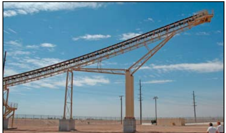
Figure 8: Elevation view of the conveyor belt system "Head End." The truss system inclines to 70 feet above grade to stockpile material.
