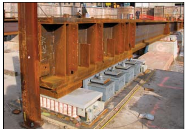
Figure 4: 1 st floor transfer girder with isolator and anchor assemblies – reaction block.
