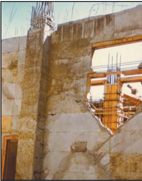
Figure 3. pre-drilling through a layer of "cemented sands" for foundation pile installation. The contractor's equipment could not penetrate the layer. The Owner (Government) offered no direct help or advice, just pointed to the soil borings logs and insisted there was no differing site condition. The contractor completed the project nine months late. He then filed a "Differing Site Conditions" claim for direct costs of $1.5 million and prepared an additional claim for acceleration costs of $5.0 million. The Owner counter-claimed $2.7 million for liquidated damages. Total claims: $9.2 million. During the Board of Contract Appeals hearing, both sides learned that there were discrepancies in the field logs. Although the Owner "won" the case, there were no real winners, only losers. In retrospect, the Owner should have been more open to the possibility of a differing site condition and considered sharing the cost of more suitable equipment. This would have been a small fraction of the cost of litigation, preparation for the court hearing, schedule delays, and the claims themselves. (Murray Walter, Inc. 1987).
