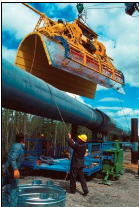
Construction of the Trans-Alaska Pipeline in the 1970s. Courtesy of Alyeska Pipeline Service Company.
