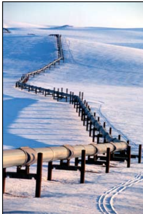
Trans-Alaska Pipeline in the winter. Courtesy of Alyeska Pipeline Service Company.
