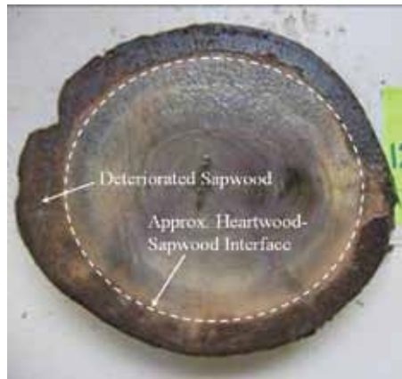
Figure 1: Deteriorated timber pile cross-section.
