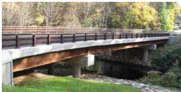
The Vernon Avenue Bridge project serves as an example of how to successfully instrument a structural health monitoring system during the construction process.
