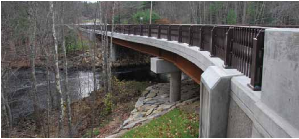
The Vernon Avenue Bridge in Barre, Mass., was one of the first “work horse” bridge projects in the U.S. to involve implementing a structural health monitoring system.
