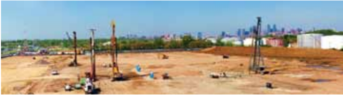
CMC Installation at the Essington Warehouse Site. Multiple rigs were on site to accelerate the construction schedule.
