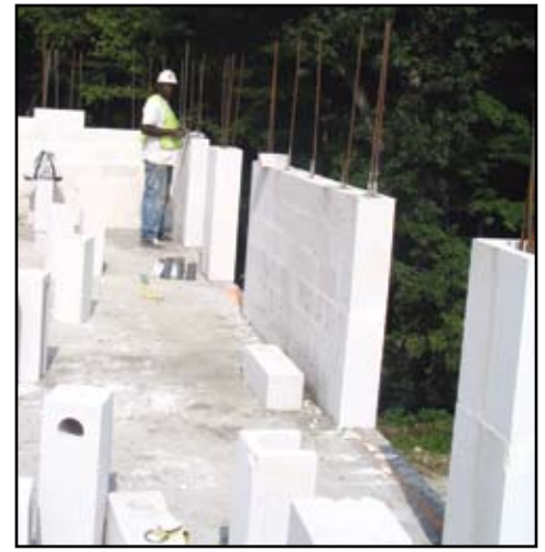
Installation of AAC reinforced block walls at State University of New York at Stony Brook.
